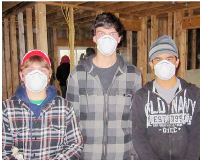
Pine Ridge Outreach Trip: Protecting ourselves from drywall dust. View additional photos on page 6
